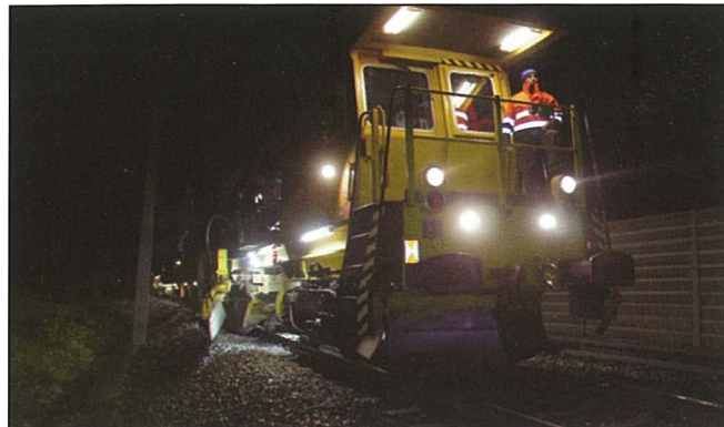
Fig. 7: The BDS 2000 performing deep sweeping on ÖBB, in order to prevent ballast flying (WN)
