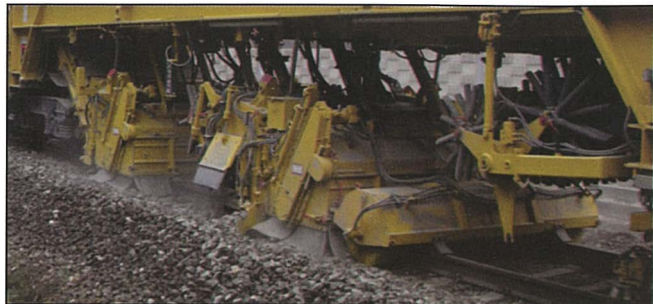
Fig. 6: The high-capacity sweeper unit of the BDS 2000 ballast distribution and profiling machine
